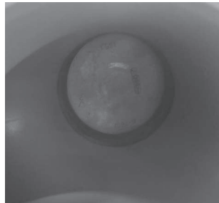
Bypass Valve Closed (Entering Water Connection)
