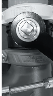
Valve Stem Position – Bypass Valve
