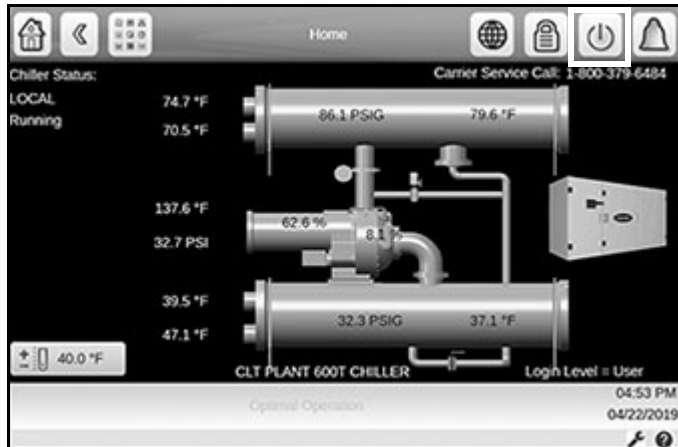
Fig. 14 — Chiller Start/Stop Icon
