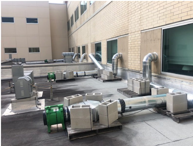
Photo 3: Single patient room negative air configuration through exterior windows. Air is exhausted by HEPA filtered air at roof level. Photo Courtesy of Orlando Health, Southlake Hospital, Orlando, Florida
