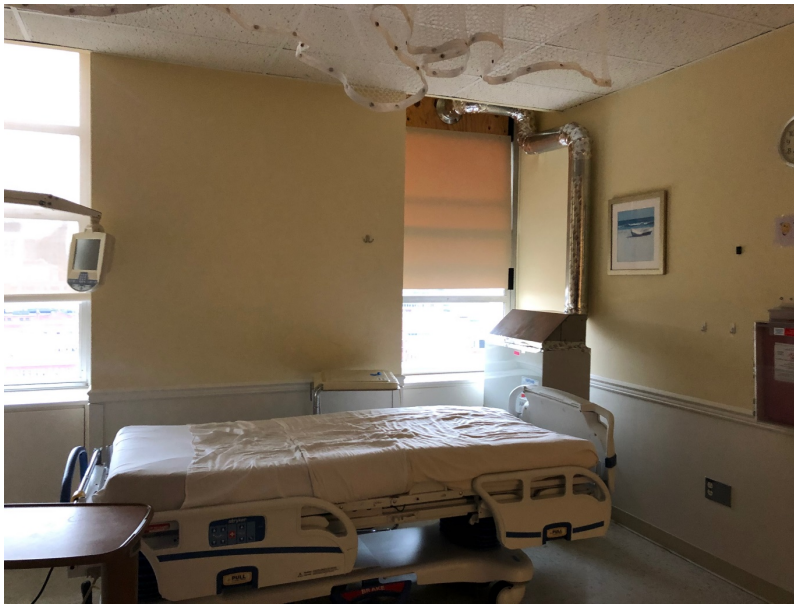
Photo 1: Temporary AIIR negative isolation room. Air is exhausted by HEPA filtered air outside.
