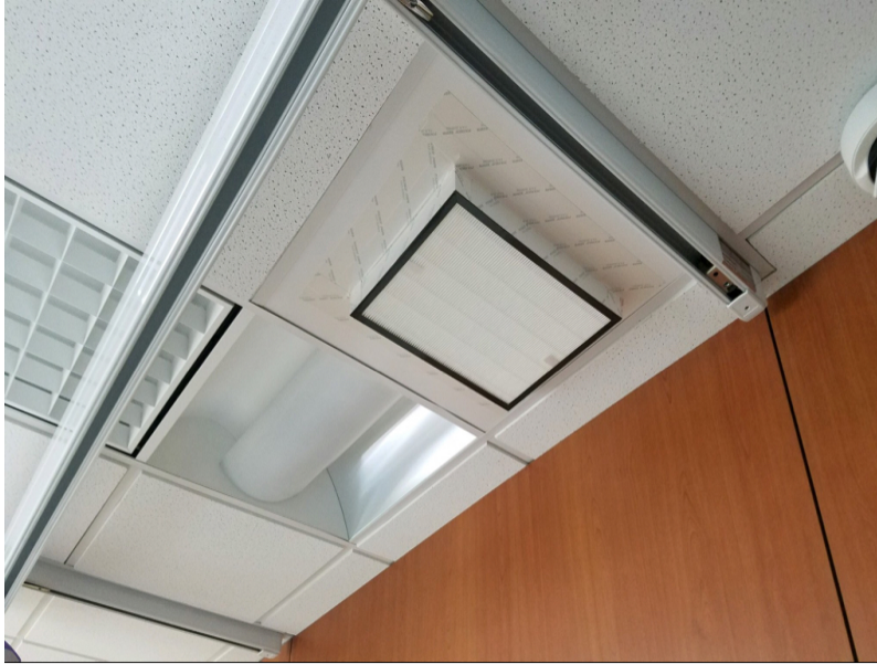
Photo 2: Installation of HEPA filter on return air diffuser in order to create temporary neutral/negative pressure for single patient room. Photo Courtesy of Naval Hospital Camp Pendleton, Camp Pendleton, California
