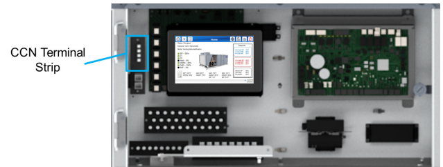
Fig. 3 – 48/50V CCN Terminal Location
