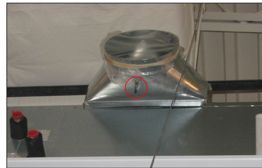
Figure 19 — Pressure Tap at Primary Air Inlet to the Induction Beam
