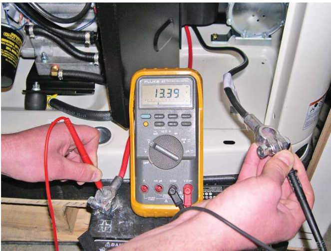
Figure 3.12 — Measurement of Charger Output with Battery Disconnected
