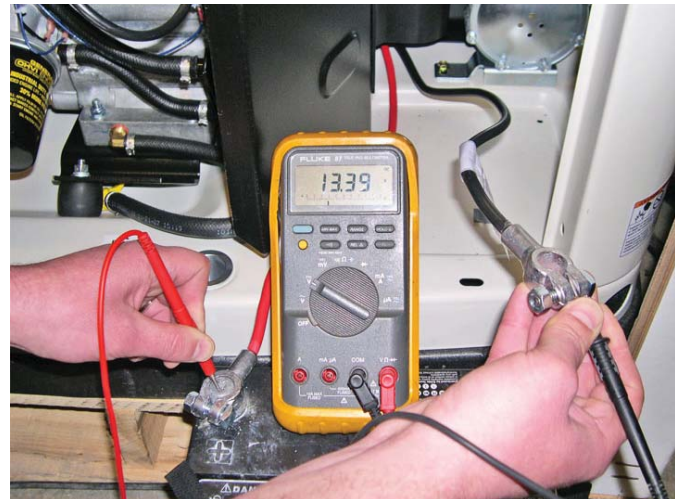
Figure 4.8 — Measurement of Charger Output with Battery Disconnected
