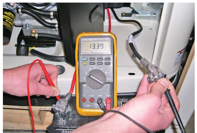
Figure 2.3 — Measurement of Charger Output with Battery Disconnected
