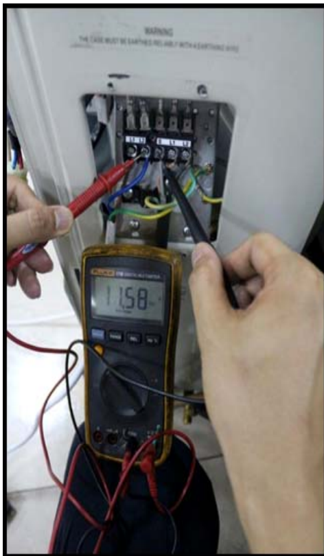
Fig. 30 – Test the DC Voltage
