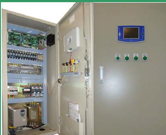
16DE PD5 CONTROL CENTER
