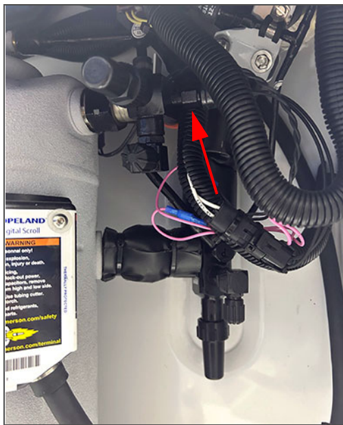
Figure 3.25 High Pressure Switch (HPS)
